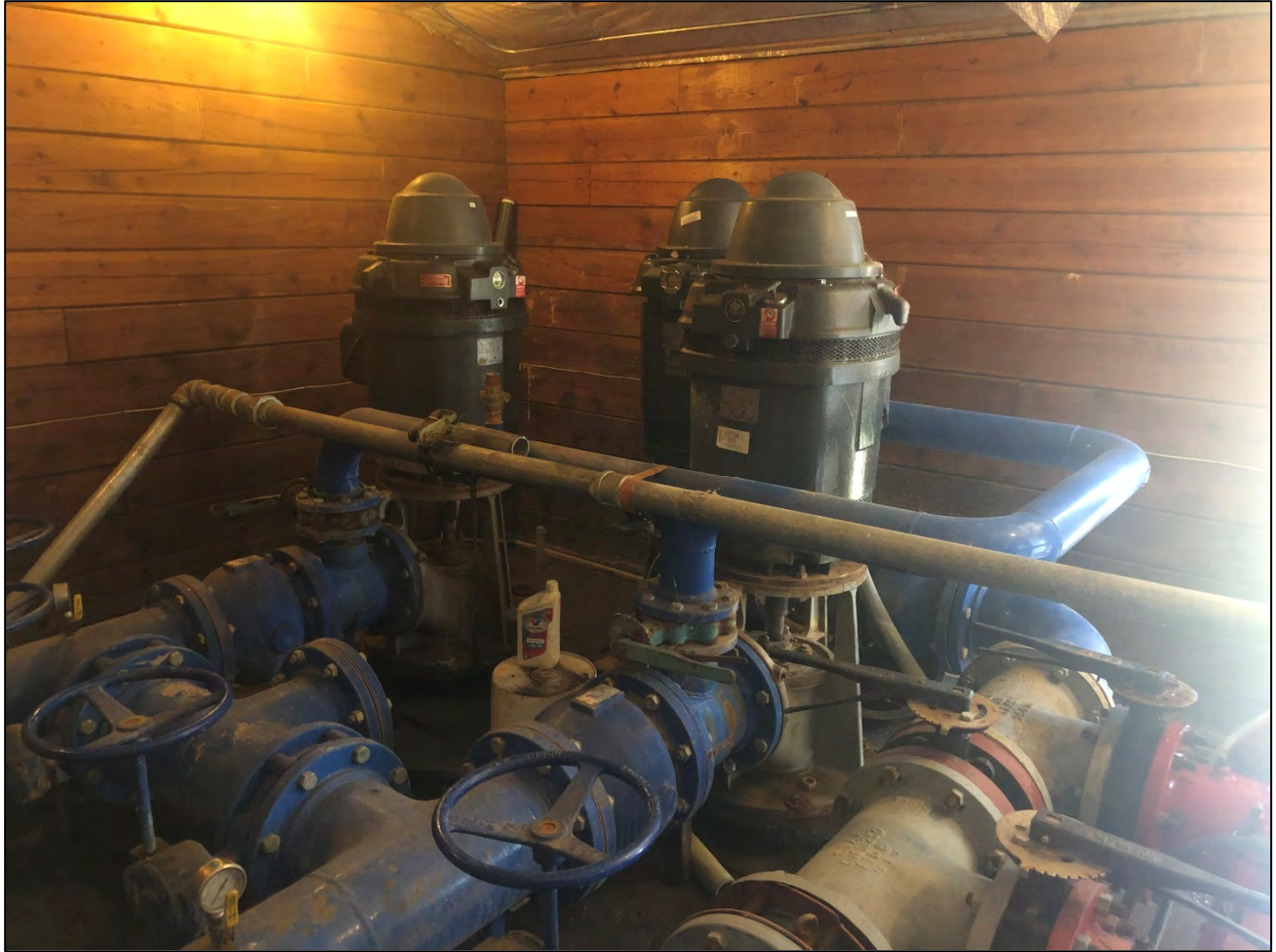
Figure 2-2. Interior of the Eagle River Pump Station
