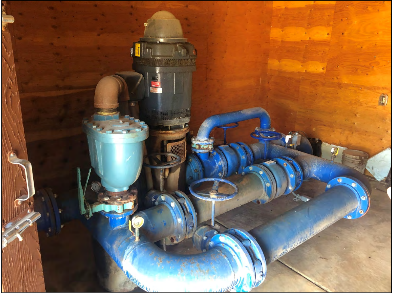
Figure 2-3. Interior of the Midway Pump Station
